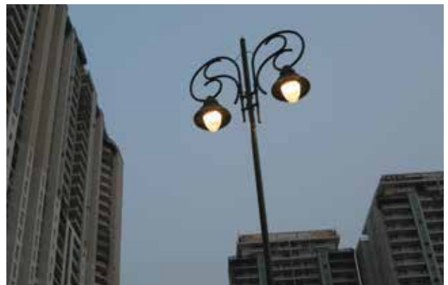
HAT FYZT-501 suspended fixture at DLF Crest (Gurgaon)
